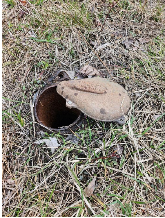
Photo 10: Unsecured well ERT-08
