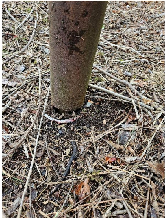
Photo 6: Damaged/corroded casing at base
