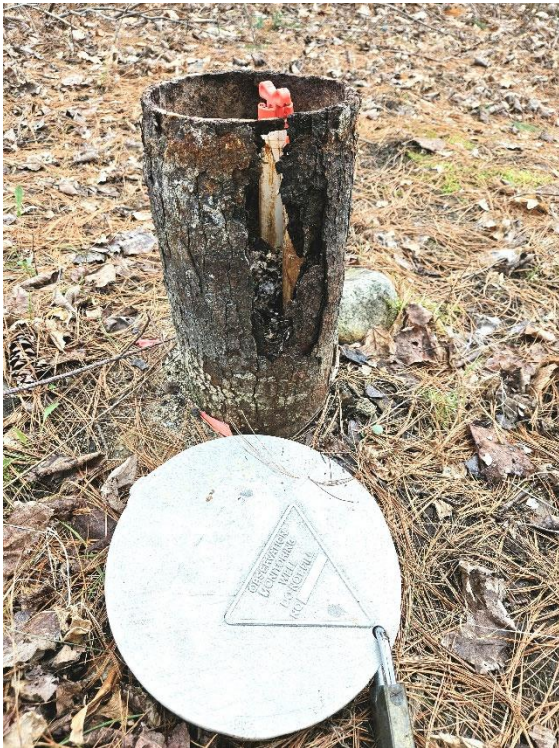
Photo 7: Severely corroded casing
