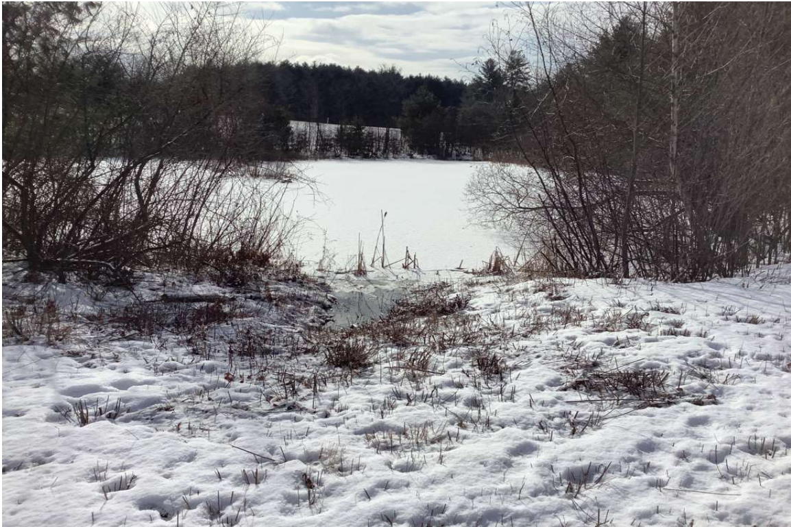
Photo No. 7: Culvert Inlet, heavy vegetative build-up at inlet removed by Town (View: South)
