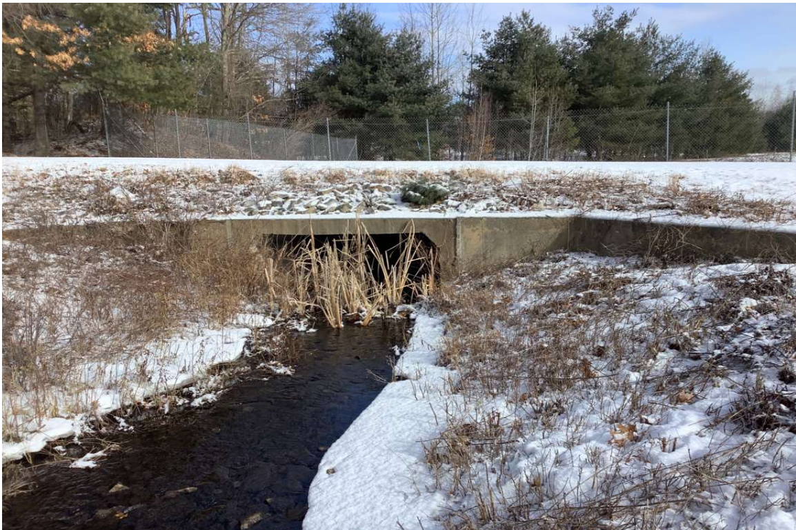
Photo No. 5: Box Culvert at Swale F, vegetative build-up at inlet (View: North)
