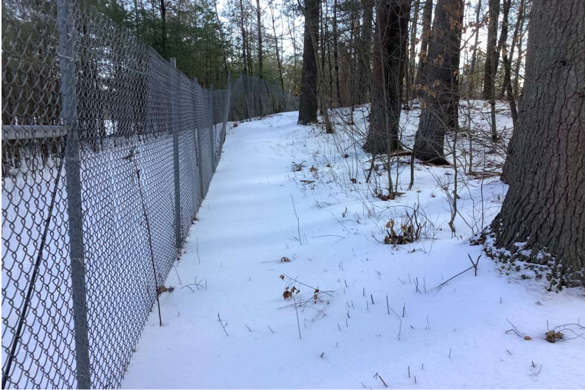
Photo No. 16: Town Dump Fence, vegetation thinned by Town (View: East)
