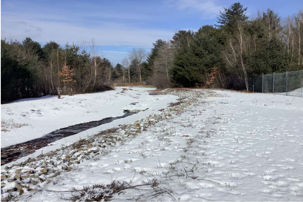
Photo No. 10: Swale C, sediment and vegetative build-up removed by Town (View: Northwest)
